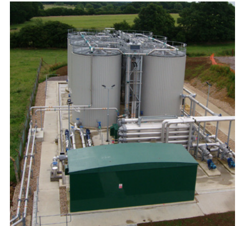
Above: A 9,700tds/annum advanced sludge digestion plant with fully integrated CHP, improving the quality of sludge and maximising biogas for energy generation. (Courtesy of Monsal Ltd.)
