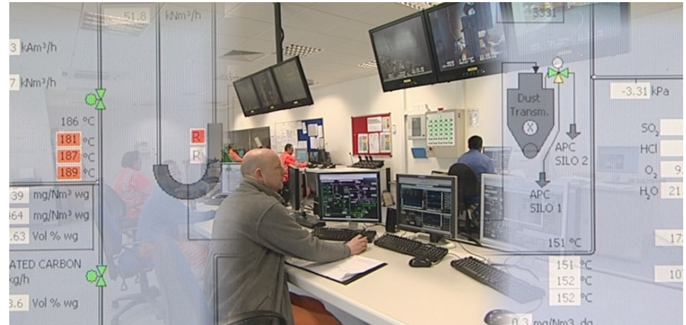
Above: Lakeside Control Room.
