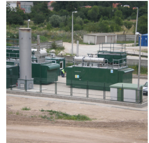
Above: Ener-G Landfill gas extraction plant at landfill site in Hungary.
