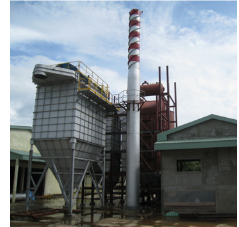
Above: New 2MWe rice husk combustion plant in Cambodia. (Courtesy of Torftech Ltd.)
