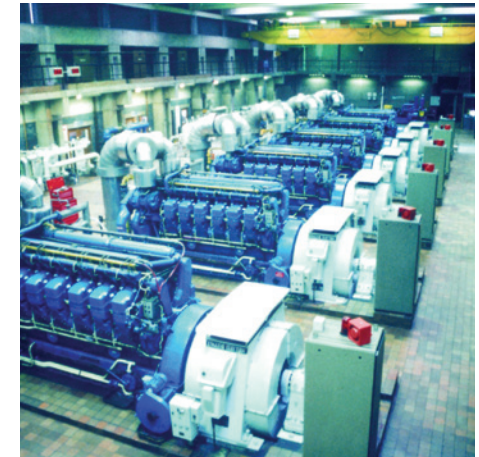
Above: A 9940kW of state of the art installed capacity, generating electricity from sewage gas from a population of one million in England's second largest city, Birmingham. (Courtesy of Monsal Ltd.)
