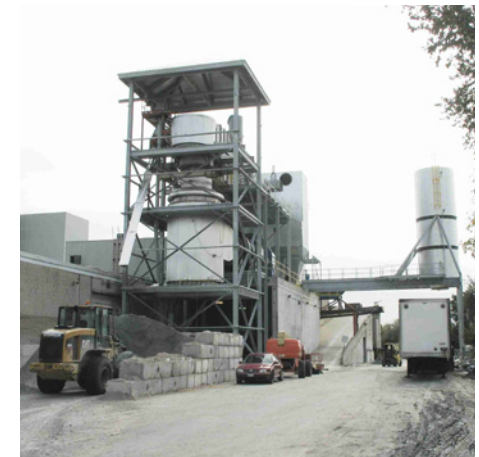
Above: 12MWth 6.0 tph Paper Sludge Combuster, Canada.
