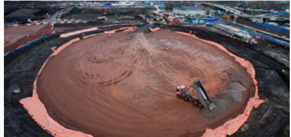
Above: Creation of building platform for London 2012 Olympic Stadium on recovered land.
